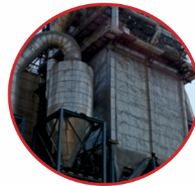
Vertical Cross Flow with Finned Tubes for AQC.
